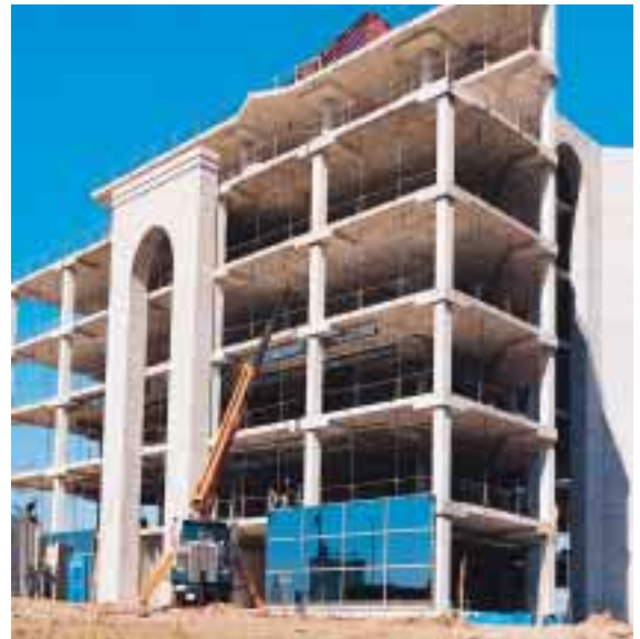
Office tower plumbed with PVC DWV pipe and fittings Courtesy IPEX, Toronto, Ontario
