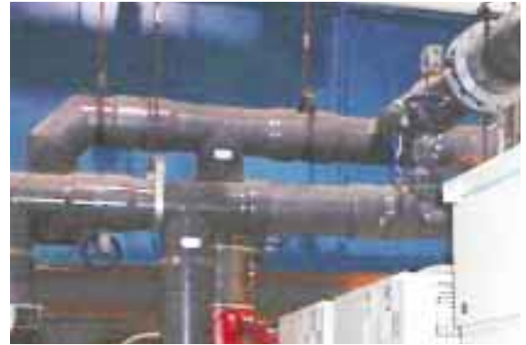
PVC Schedule 80 pipe is used in a pressure application in Freedom Plastics' chiller room. Courtesy Freedom Plastics, Janesville, Wisc.
